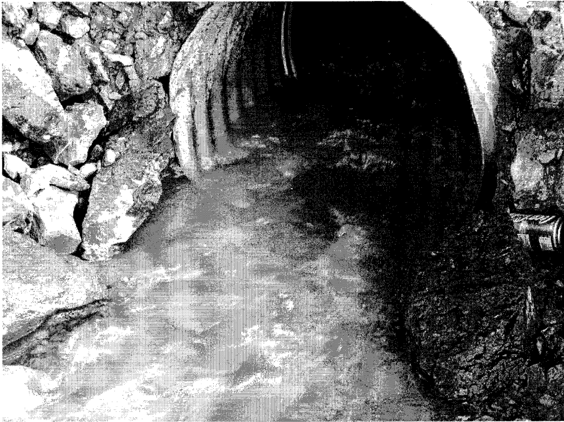
Photo 2: Inlet channel leading to overflow culvert at Tailings Pond no.1. Note the absence of adequate protection from erosion other than backfill with material excavated from the dam itself. Also note the use of an old and corroded 24-inch corrugated steel pipe.
