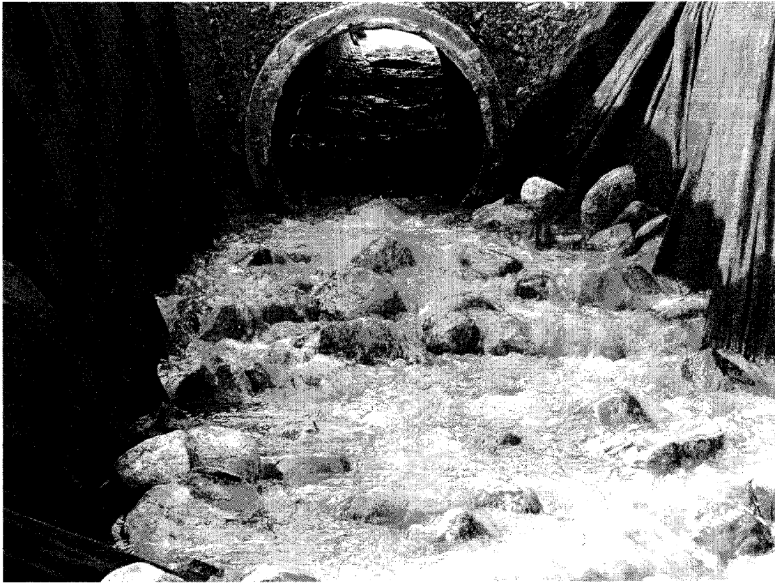
Photo 3: Outfall channel from overflow culvert at Tailings Pond no.1. Note the absence of adequate protection from erosion other than a poorly anchored geotextile under which water was observed flowing. Also note the erosion on the left side, between the geotextile and the wall of the old 24 –inch concrete pipe. Given the rudimentary installation of the culvert and the quality of materials used, it is likely that the joint between the corrugated steel and concrete culvert sections is not watertight, and that water infiltration at this location is mining the dam from the center out.
