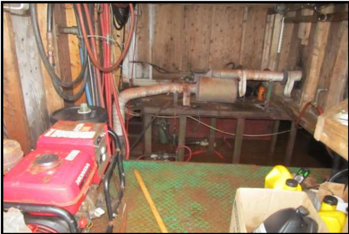
MACHINERY SPACE BELOW WHEELHOUSE – LOOKING STARBOARD
