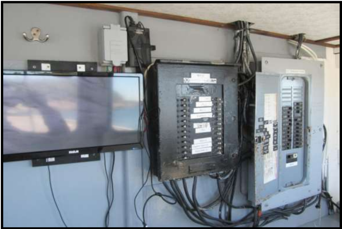
VESSEL ELECTRICAL PANELS LOCATED IN WHEELHOUSE
