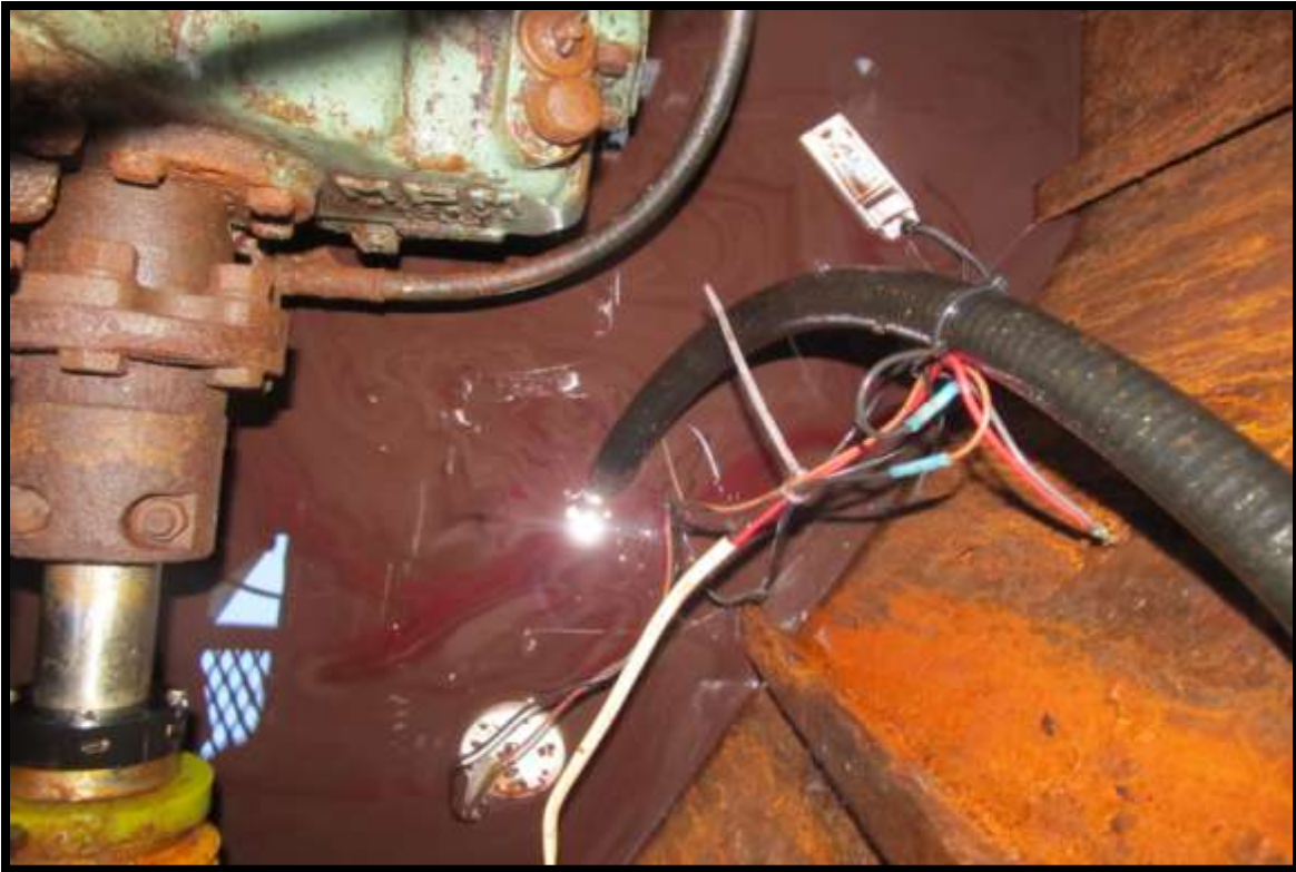
ENGINE ROOM BILGE PUMP
