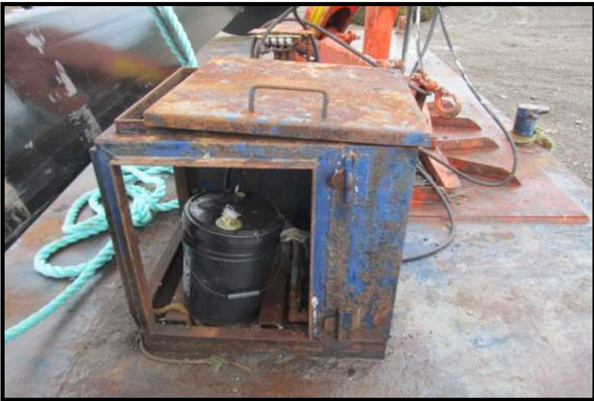
ENCLOSURE FOR HPU – NOT INSTALLED
