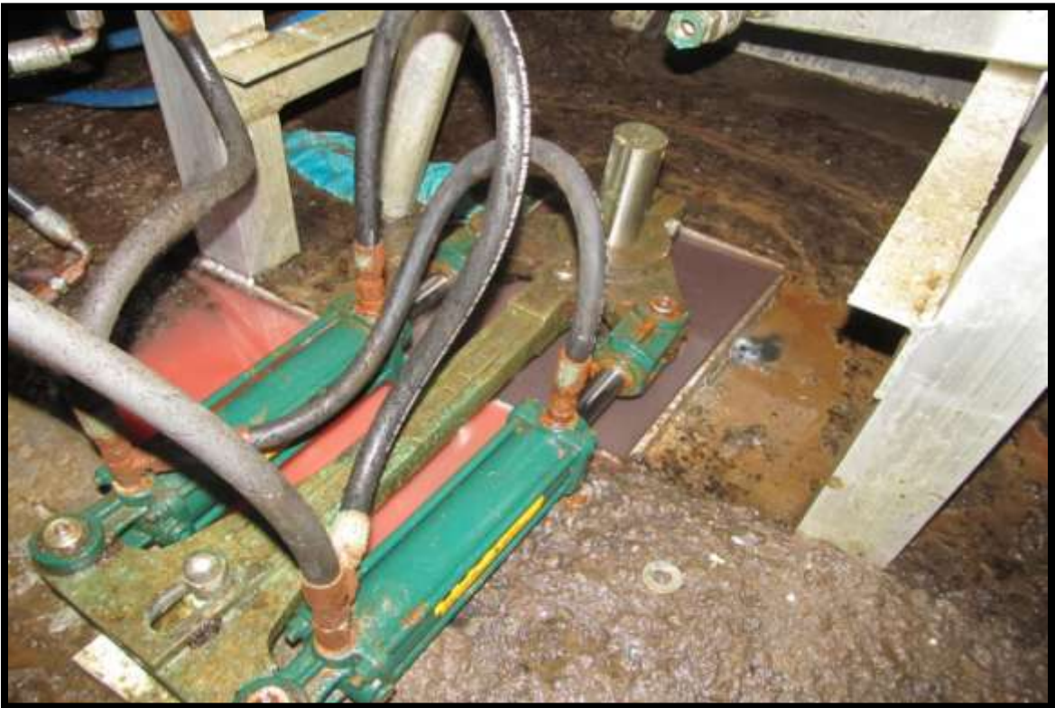
STEERING GEAR – AFT VESSEL COMPARTMENT
