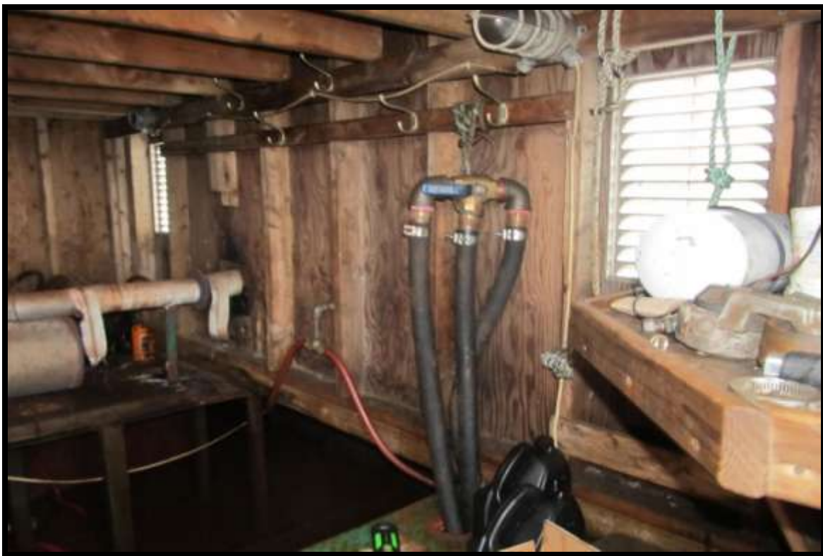
MACHINERY SPACE BELOW WHEELHOUSE – LOOKING AFT
