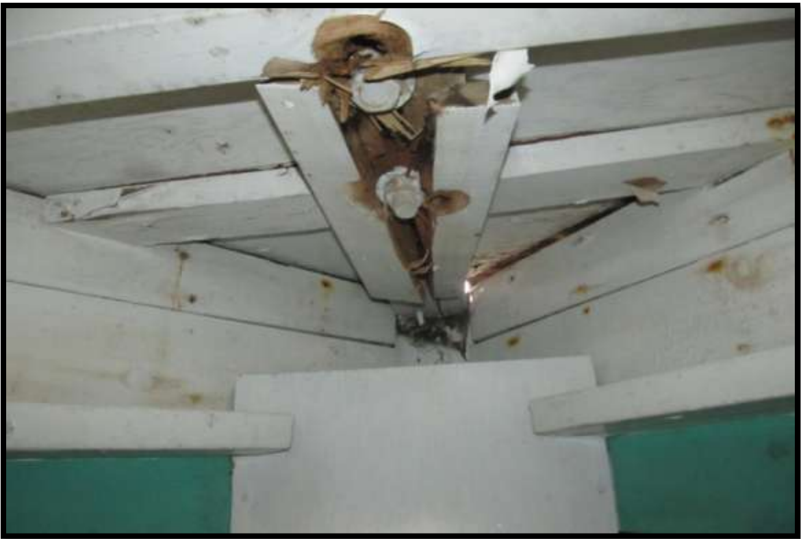
FOC'SLE DECK STRUCTURE DAMAGE
