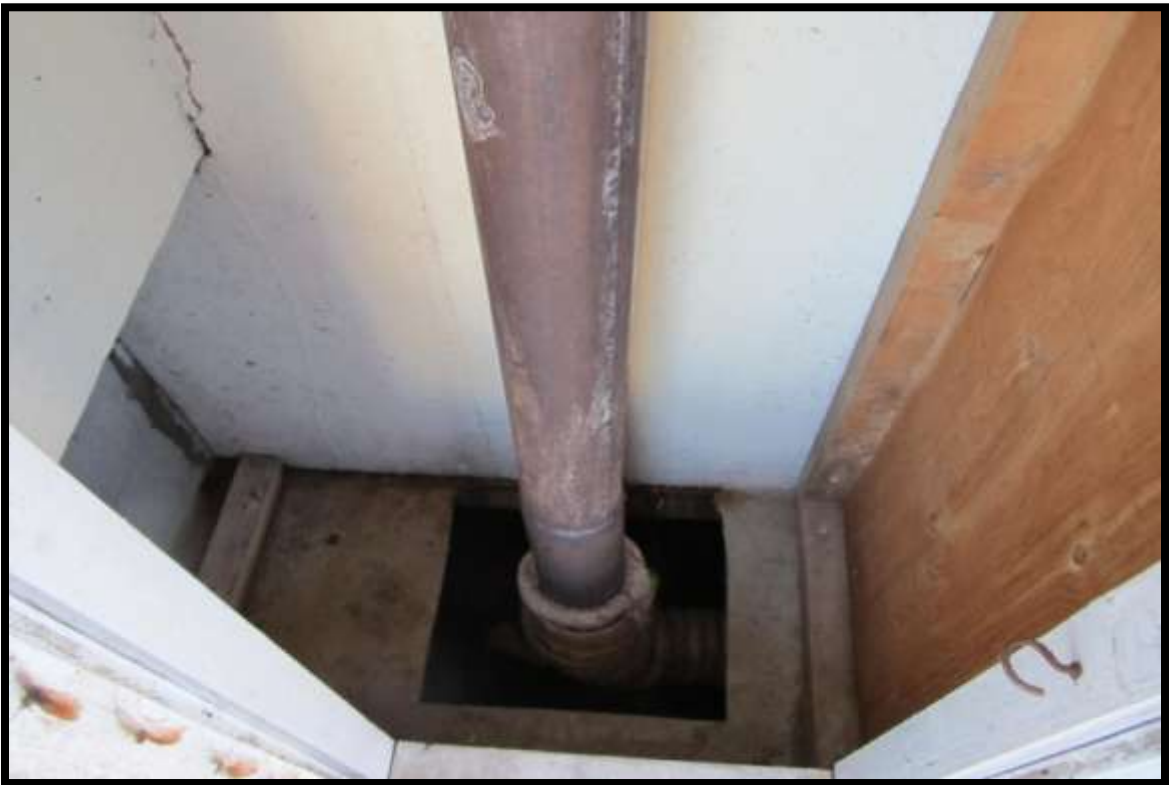
ENGINE EXHAUST – MAIN DECK PENETRATION
