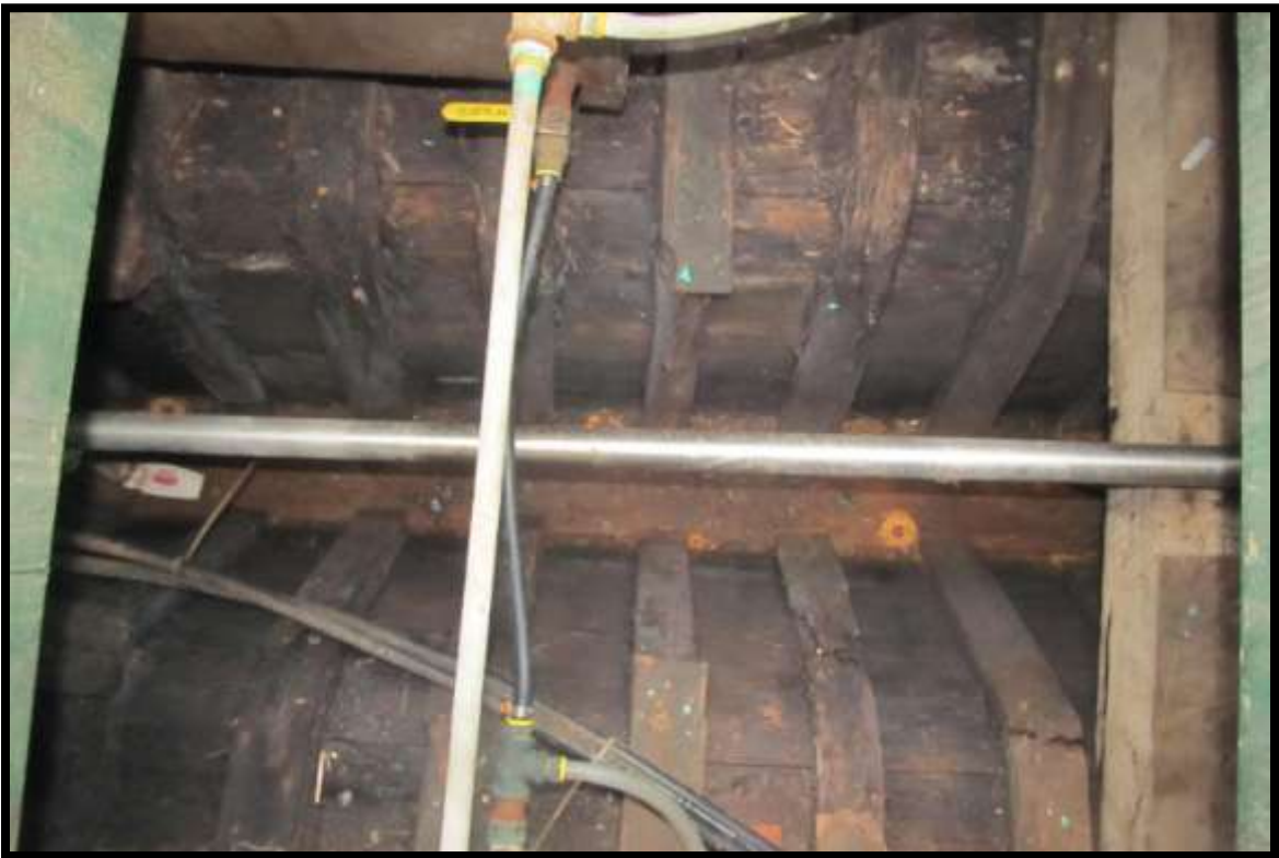
SHAFTING/HULL STRUCTURE IN WAY OF FUEL TANKS
