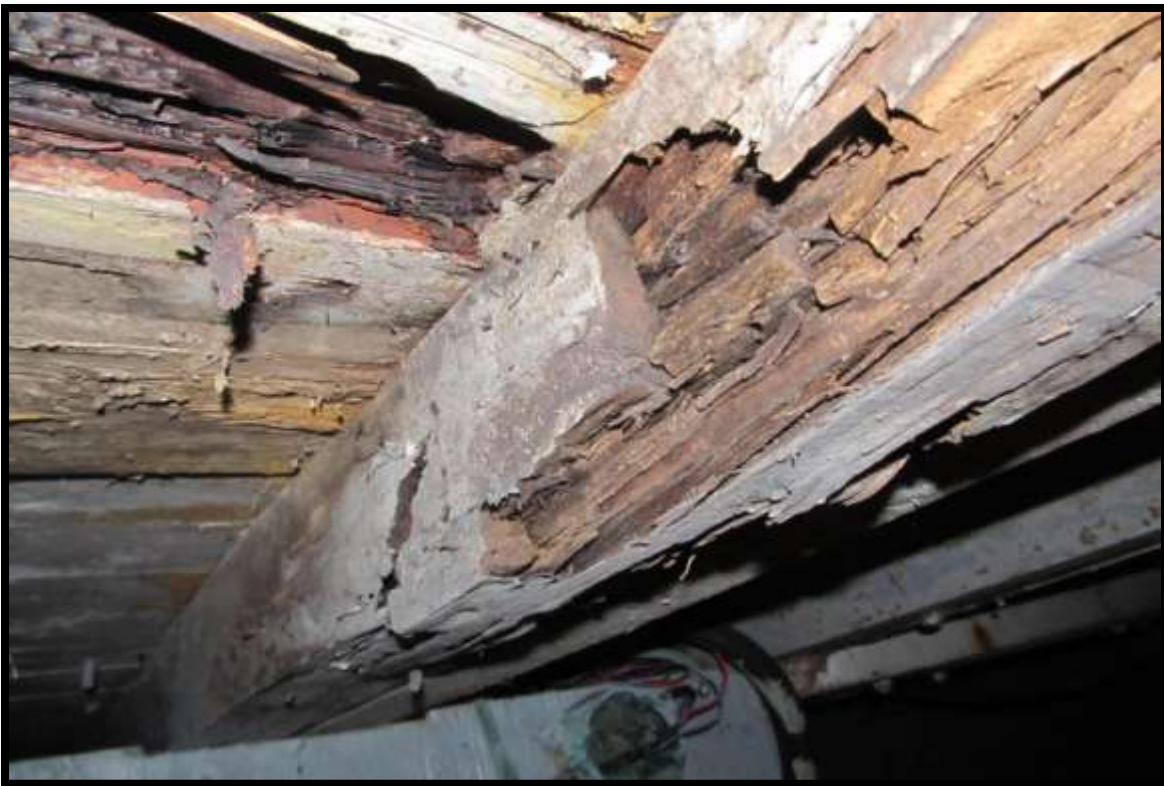
MAIN DECK STRUCTURE WITHIN FISH HOLD. EXTENSIVE ROT NOTED
