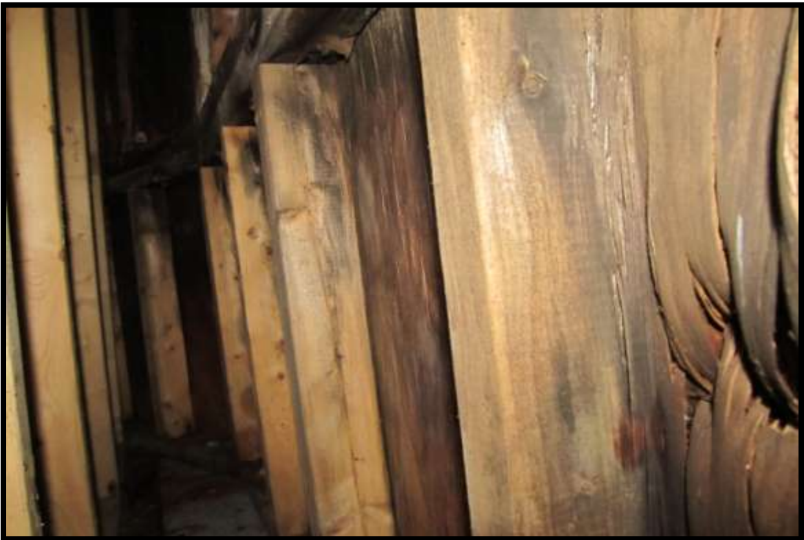
WHEELHOUSE FRONT STRUCTURE. EXTENSIVE ROT NOTED
