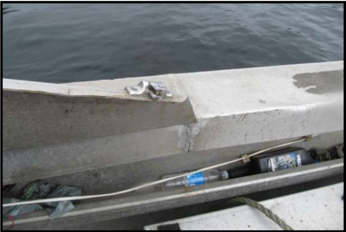
BULWARK WELD FRACTURE
