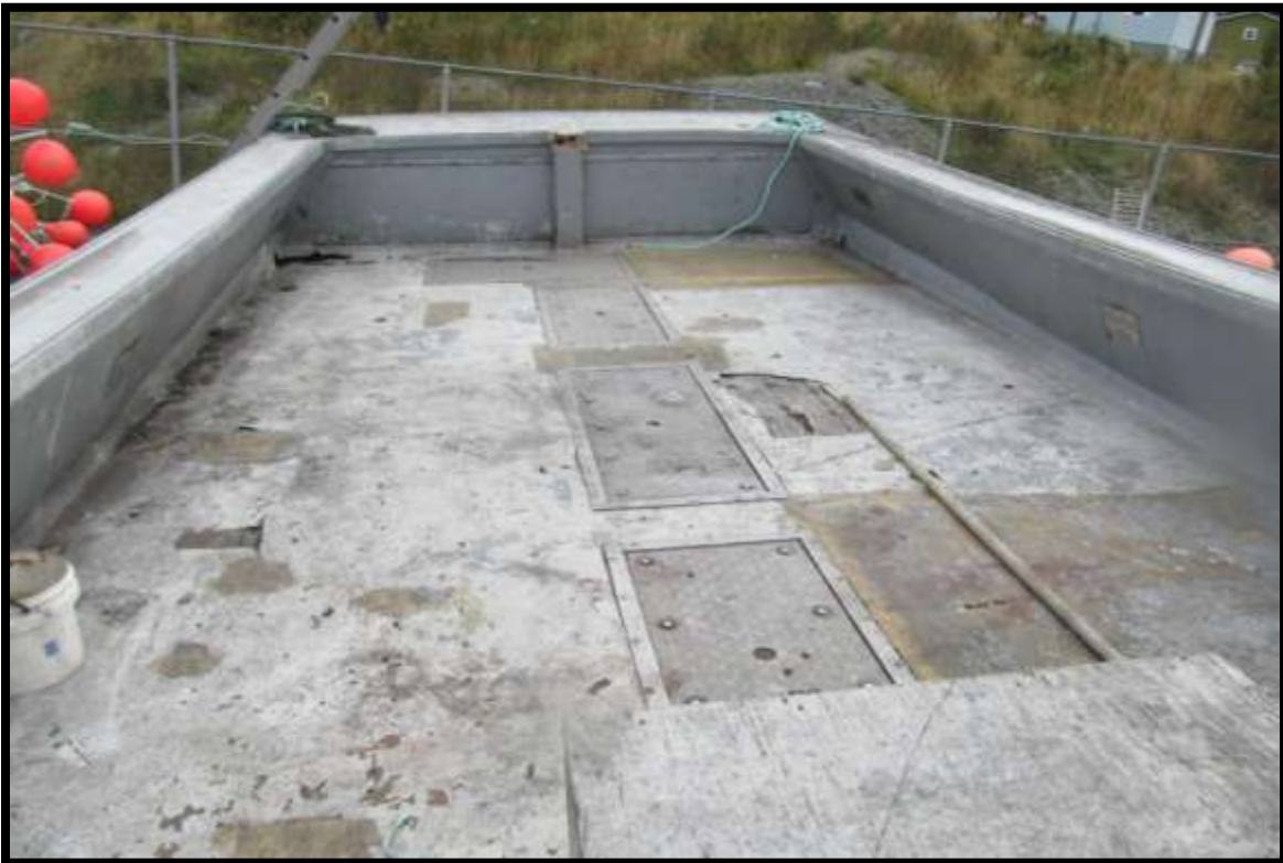
MAIN DECK LOOKING AFT. EXTENSIVE DELAMINATION NOTED
