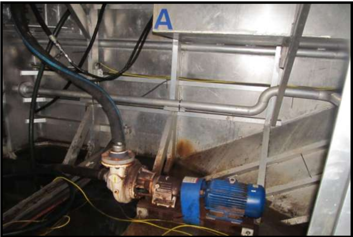
SEAWATER PUMP FOR FEED SYSTEM
