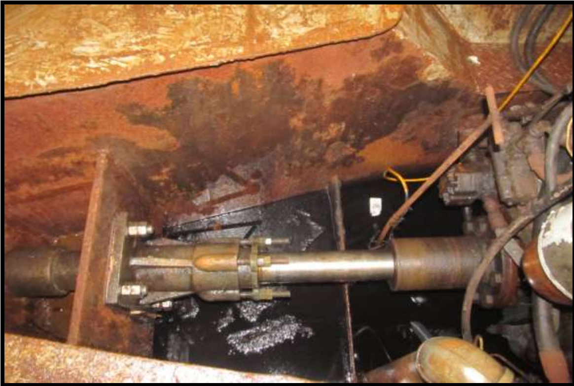
TAILSHAFT, SHAFT SEAL AND BEARING
