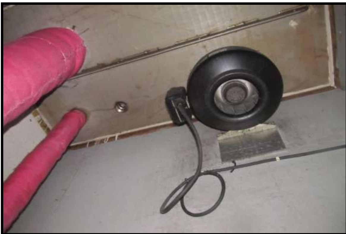
EXHAUST CASING LOOKING UP
