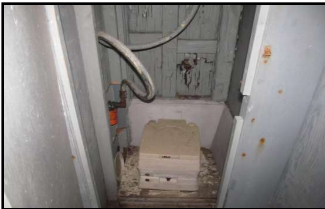
MAIN DECK WASHROOM. EXTENSIVE ROT NOTED
