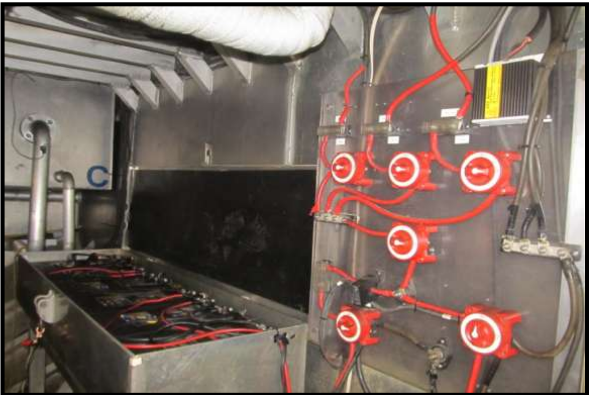
BATTERY BOX AND SWITCHES
