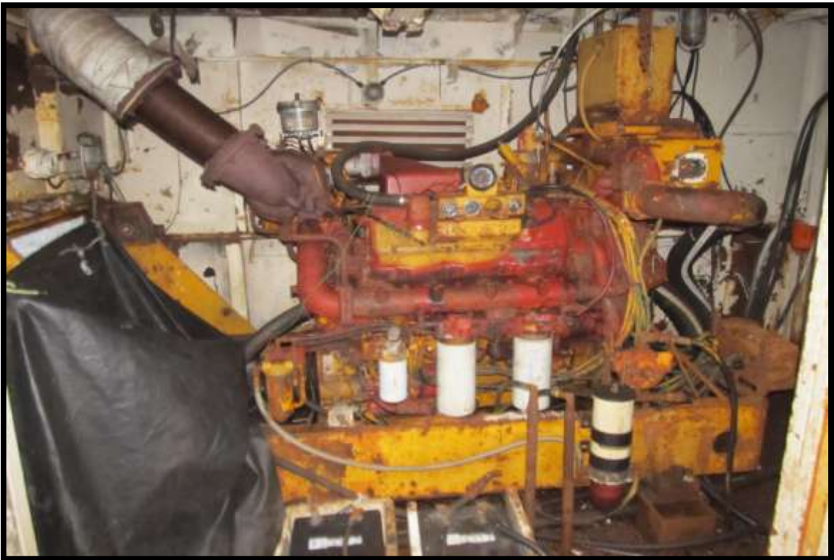
AFT MAIN ENGINE
