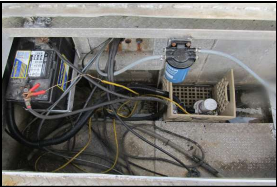
BATTERY, FUEL FILTER AND BILGE PUMP
