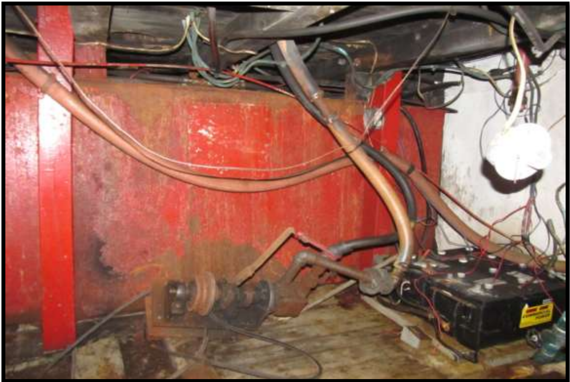
ENGINE ROOM COMPARTMENT LOOKING STARBOARD
