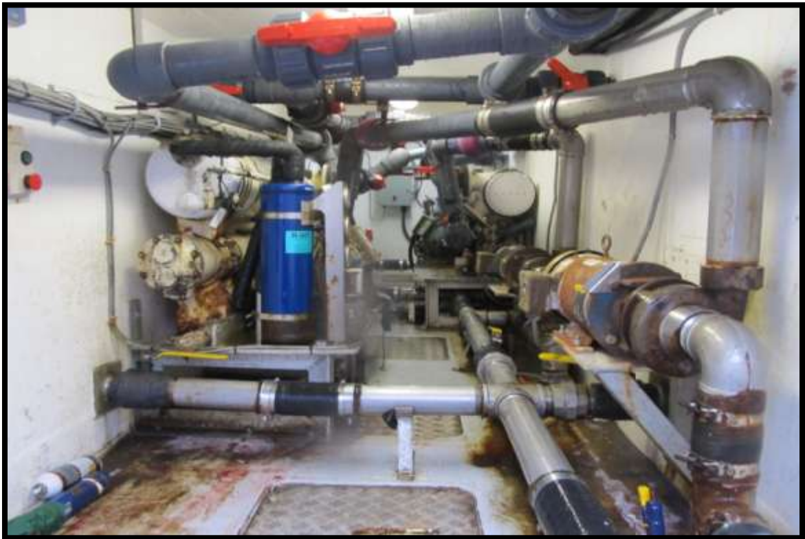
RSW EQUIPMENT LOCATED BETWEEN RSW TANKS
