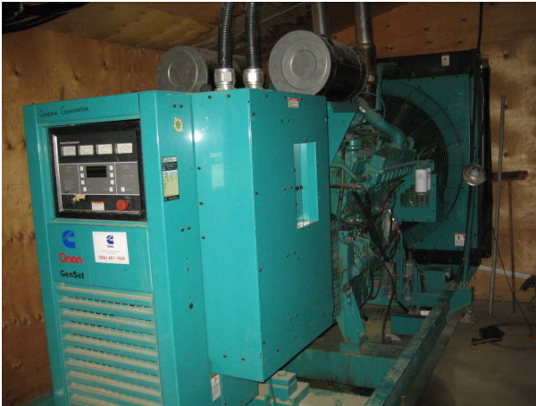
Ref. #62 Cummins Model DFGB-3370073, 600-KW Diesel Generator, S/N D990897895 (New 1999)
