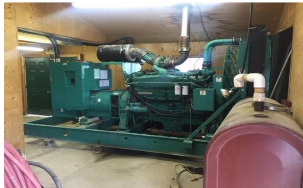
900hp Diesel Generator
