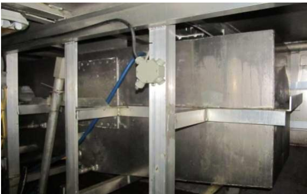
Fuel Tank (Aft Vessel Compartment)
