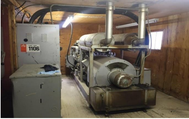
500hp Diesel Generator
