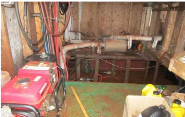
Machinery space below wheelhouse
